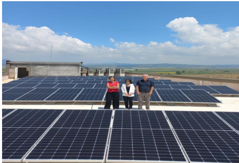
Figure 10 . Yumurtalık Vocational School Solar Power Plant
