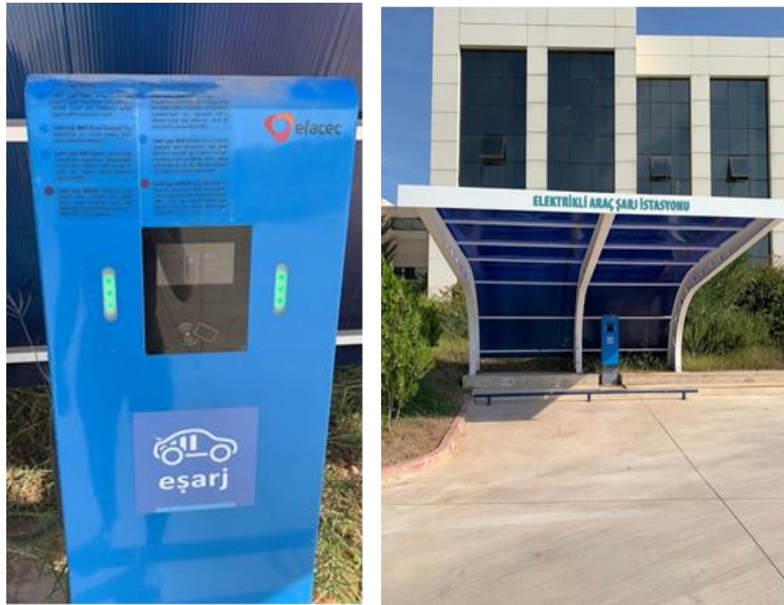
Figure 27. Charging station for electric vehicles
