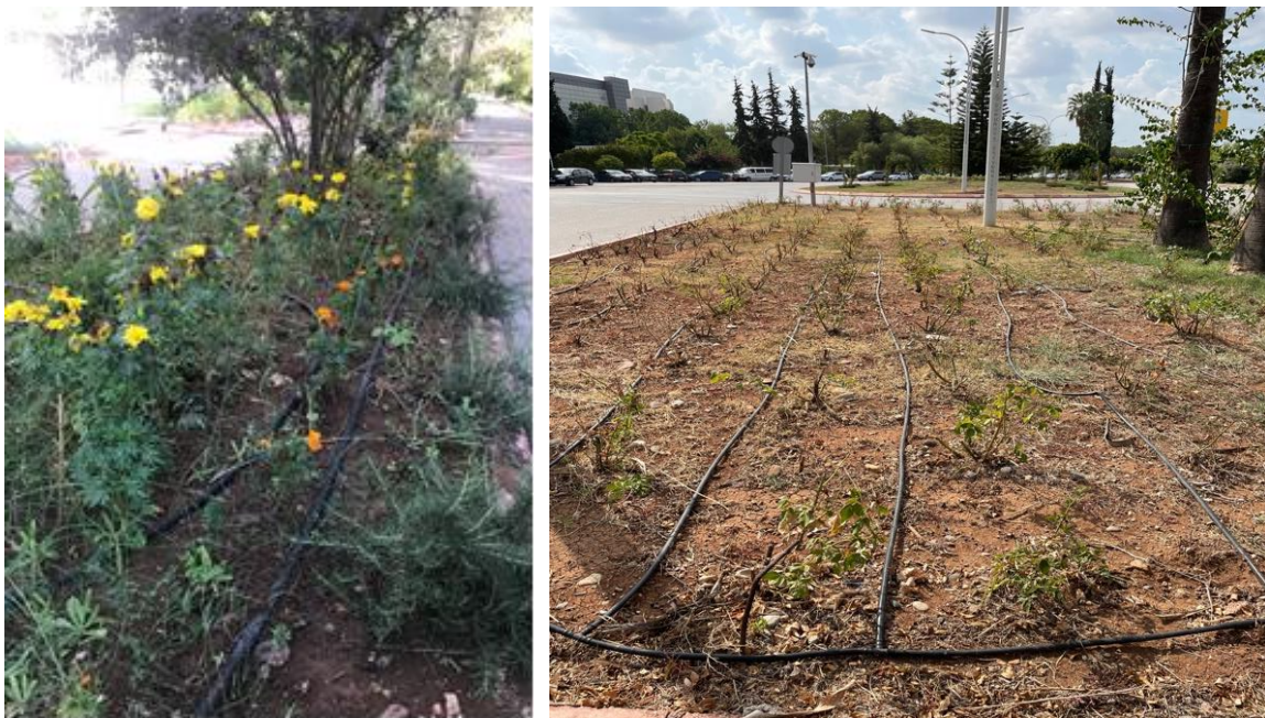
Figure 22. Drip Irrigation System
