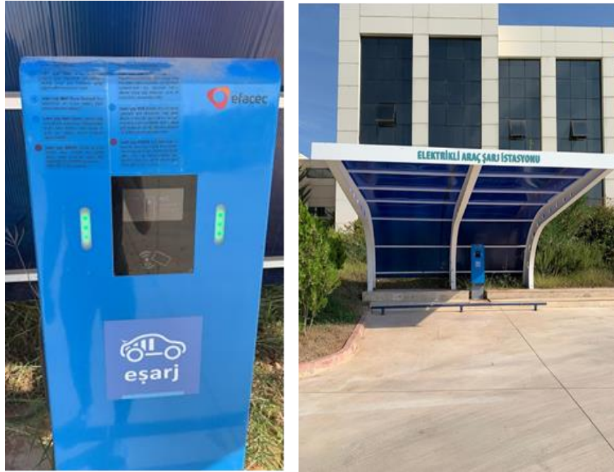
Figure 27. Charging station for electric vehicles
