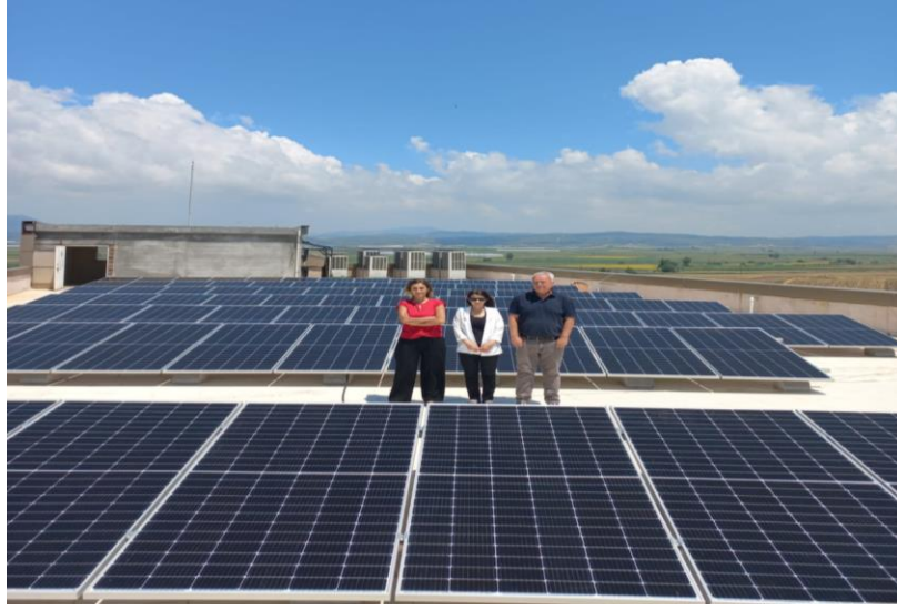
Figure 10 . Yumurtalık Vocational School Solar Power Plant
